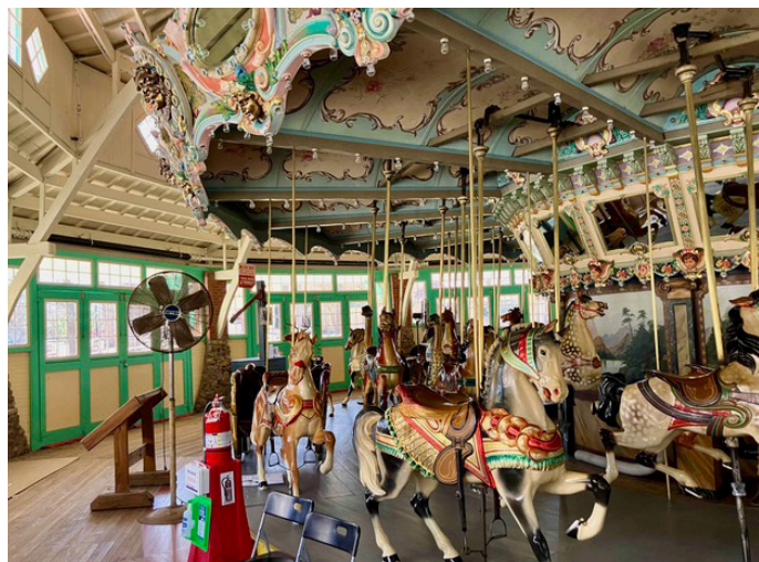
Concealed sprinklers protect the inside of Glen Echo Park Carousel.
